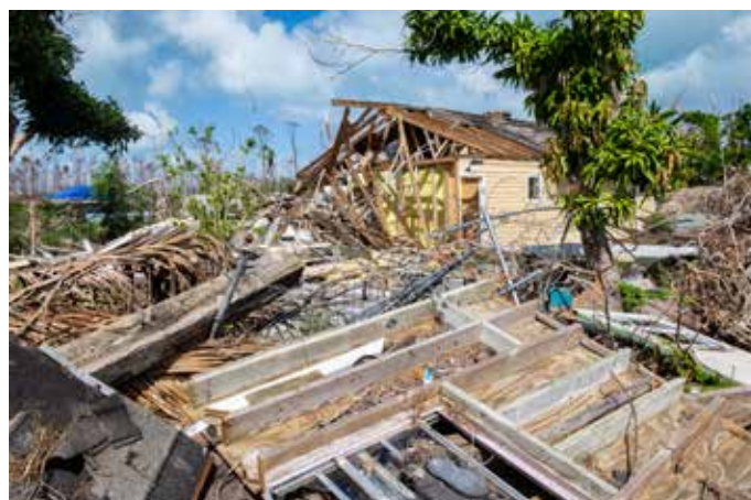
Fig. 13. Destroyed houses in Marsh Harbor on Great Abaco Island after Hurricane Dorian swept by on September 5, 2019. Photo: Shutterstock
